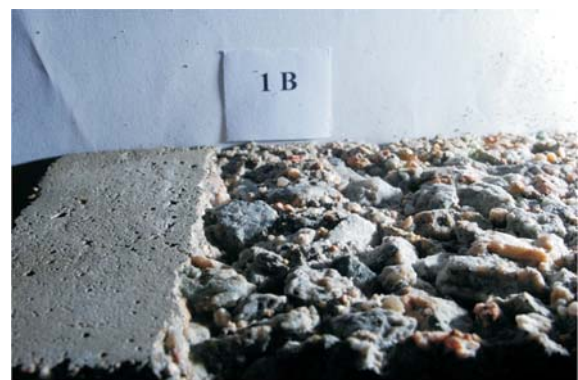
Figure 2 C 20/25 concrete, transition between uncurved concrete surface (left) and blasted concrete surface (right), pressure 210 MPa
