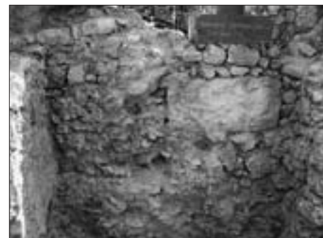
SL. 10. MASIVNI KAMEN PREKO KOJEGA JE ZATEZANA SKELA, LIJEVA OBALA FIG. 10 MASSIVE STONE BLOCK ACROSS WHICH THE SCAFFOLD WAS TIED UP, LEFT BANK
