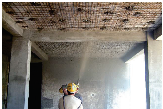
Figure 24 Repair of RC slab (additional reinforcement and executing of new concrete layer)
