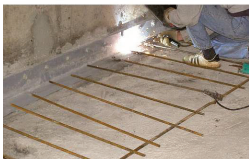
Figure 27 Execution of strengthening of RC slabs in the zone of existing RC wall
