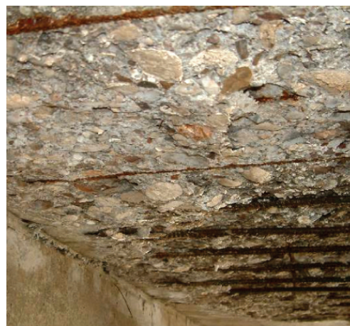
Figure 2 Severely damaged RC slab after fire
