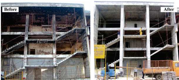
Figure 32 Changed static system of existing cantilever staircase (new RC columns and strengthened beams)
