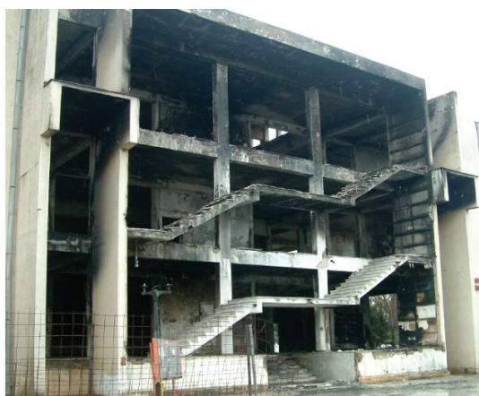
Figure 1 View of the front facade of the building after fire
