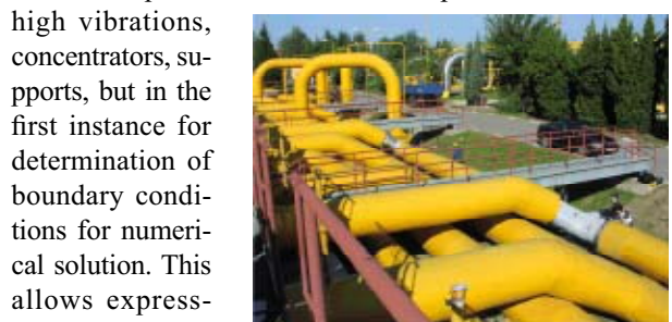
Figure 4. Location of T shape pipe on the discharge pipe chosen for stress analysis
