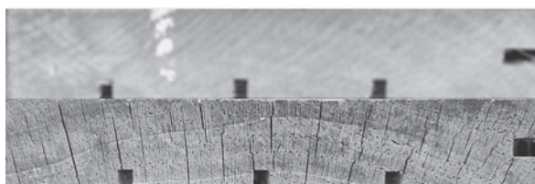
Figure 13 Furfurylated radiata pine wood deck prior to (up) and after 36 months of weathering (down)
