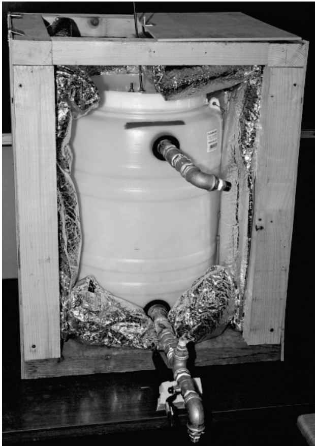
Figure 3 Storage tank – plastic barrel capacity of 60 litres – installed in box, prior to thermal insulation
