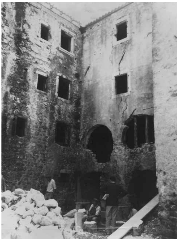
8. Nikola Vranić, Radovi na palači Vukasović, 1955. (Ministarstvo kulture RH, Konzervatorski odjel u Rijeci, Fototeka, inv. br. 17508) / Nikola Vranić, Construction works on the Vukasović palace, 1955 (Ministry of Culture, Conservation Department in Rijeka, Photo library, inv. no. 17508)
