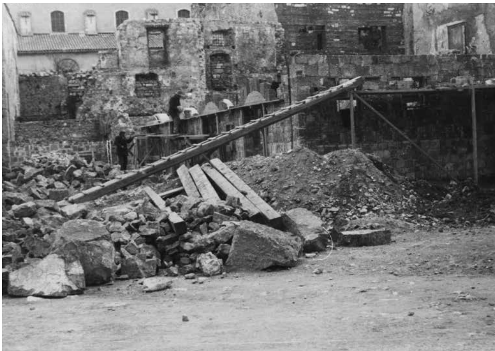
14. Fran Šijanec, Nova tržnica u izgradnji na senjskom Trgu žrtava fašizma, 1954. (Ministarstvo kulture RH, Konzervatorski odjel u Rijeci, Fototeka, inv. br. 5084) / Fran Šijanec, Construction of the new market on the Trg žrtava fašizma (Victims of Fascism Square) in Senj, 1954 (Ministry of Culture, Conservation Department in Rijeka, Photo library, inv. no. 5084)
