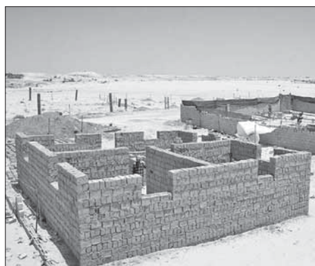
FIG. 8 EXAMPLE OF APPLICATION OF CLAY BRICK IN THE PALESTINIAN ARCHITECTURE SL. 8. PRIMJENA GLINENE OPEKE U PALESTINSKOJ ARHITEKTURI
