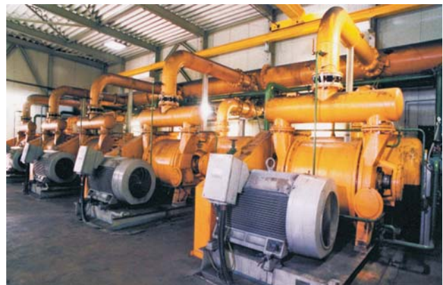
Figure 3: Degasification station. 5 units of water circle vacuum gas stations
