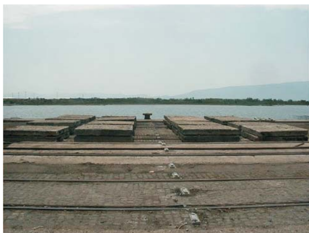
Figure 2 Loading of the harbour structure with 2 slab rows Slika 2. Opterećivanje obale s dva reda ploča
