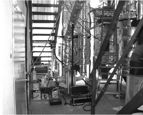
Slika 4: Sustav tretmana dimnih plinova u pilot spalionici Figure 4: Pilot incinerator flue gas treatment devices
