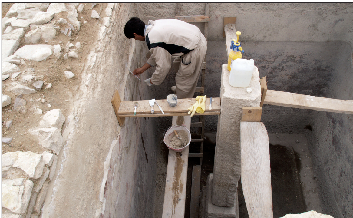
Sl. 6. Konzervatorski radovi na antičkoj cisterni u urbanom tkivu grada. Fig. 6. Conservation works at the ancient cistern in the city's urban part.
