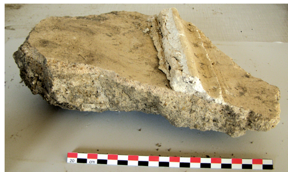
Sl. 10. Zidna žbuka s ostacima štukature. Fig. 10. Plaster with the stucco remains.
