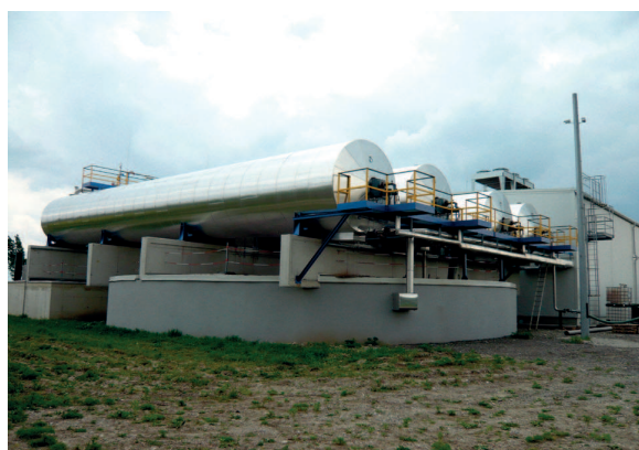
Figure 2 A view of steel tube fermenters (top) and a concrete fermenter (bottom) – BGS Zwentendorf (Austria) - photo by authors.
