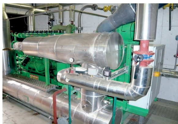
Figure 1 Cogeneration unit GE Jenbacher – photo by authors.
