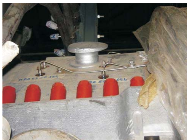
Figure 9 Pressure measurements on AE64.3A+ installed in Vlore
