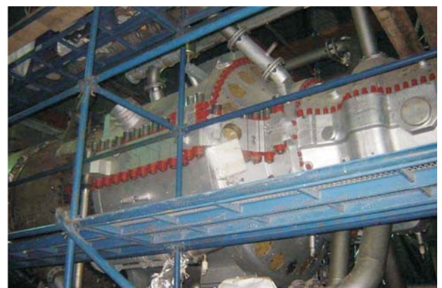
Figure 7 AE64.3A+ gas turbine installed in the Vlore site
