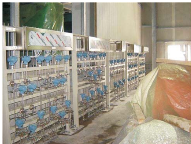
Figure 8 Instrument racks in Vlore for additional instrumentation
