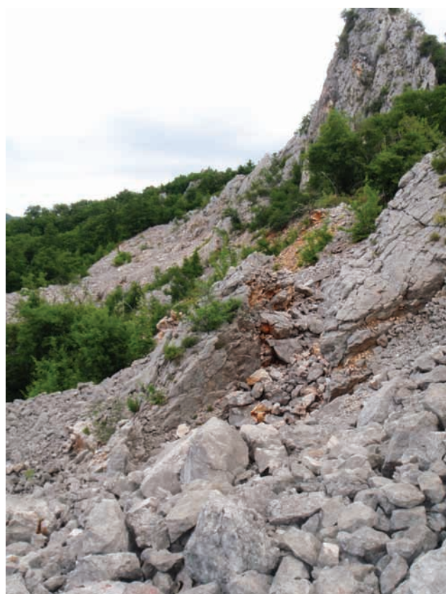
Figure 11: New open fracture on the higher eastern part of the slope (photo: BENAC, Č.).
