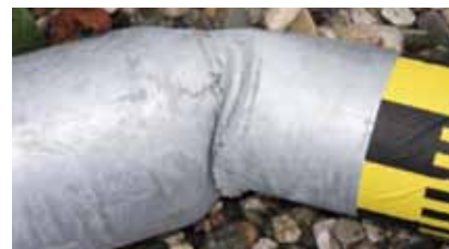
Figure 7. Column details following its fall to the ground [6]
