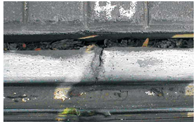
Figure 18 Damaged rail weld on tram track in Zagreb
