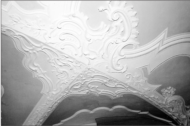
Rector's Palace, Court Hall, stucco (photograph: Katarina Horvat-Levaj)
