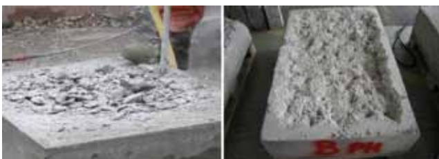
Figure 3. Pneumatic treatment (pick-hammering) of top concrete surfaces of blocks A and B
