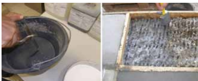
Figure 6. Preparation of binder: proportioning and manual mixing of mortar with latex marked LMC+, and rubbing into the surface of blinding concrete
