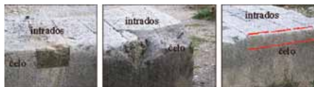
Figure 6. Some points of damage and repair on remains of demolished bridge
