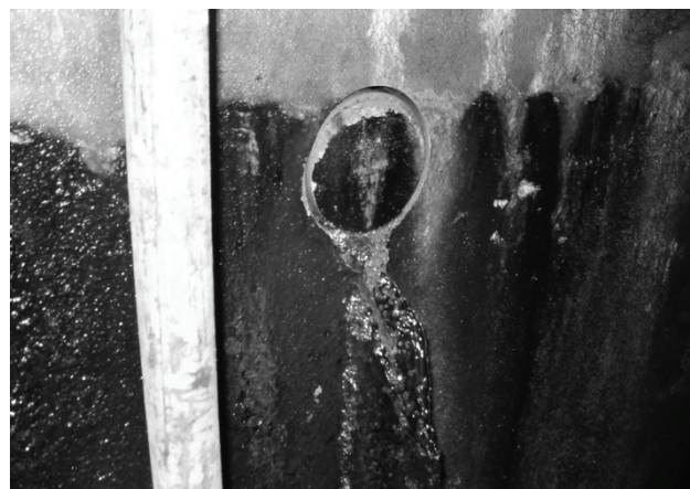
Figure 5 Water penetration at the concreting joint
