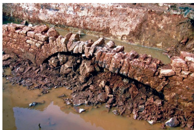
Sl. 3 Rasteretni lučni zid u unutrašnjosti vodospreme Fig. 3 The arched relief wall in the interior of the water reservoir.
