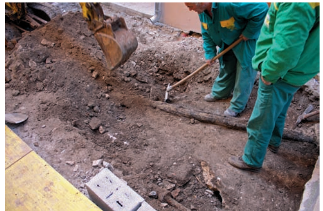
Sl.2d Pogled na kombinirani iskop u donjem dijelu Uspona Frana Glavinića (foto: R. Zlatunić) Fig. 2d A view of the combined pavement removal in the lower section of the Fran Glavinić Gradient (photography R. Zlatunić).
