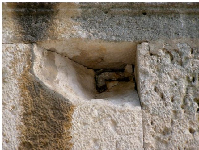
Sl. 17 Primjer željeznog klina u strukturi spomenika Fig. 17 An example of an iron spike in the structure of the monument.
