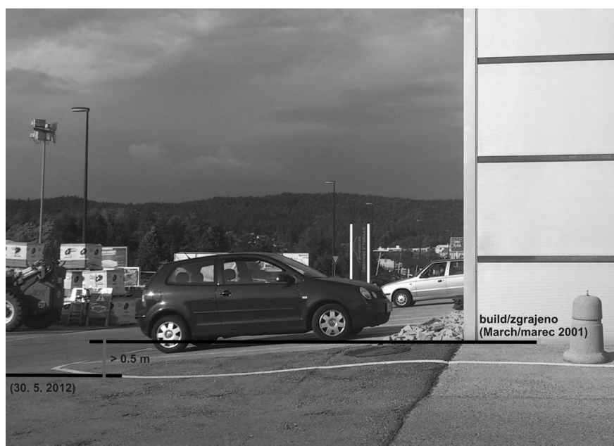
Figure 9 Subsidence at the Rudnik shopping center in southern Ljubljana (photo: David Bole). In ten years, the surface has subsided by approximately 0.5 m.
