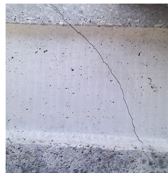
Figure 16 Shear cracks in the vicinity of supports
