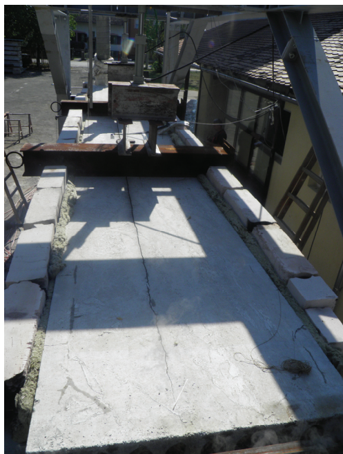
Figure 15 Test slab with a large longitudinal crack at the end of experiment
