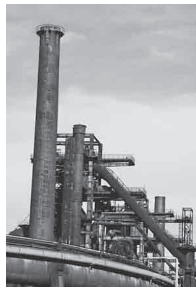
Figure 1 Effect of atmospheric corrosion
