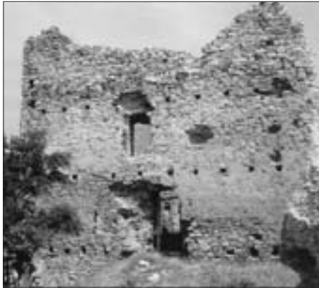
SL. 30. BURG VELIKA KOD POZEGE, JUŽNO PROČELJE BRANIČ-KULE: TRAGOVI TRIJU ETAŽA DRVENIH GALERIJA FIG. 30 VELIKA CASTLE NEAR POZEGA, DEFENSE TOWER, SOUTH ELEVATION; TRACES OF WOODEN GALLERIES ON THREE FLOORS
