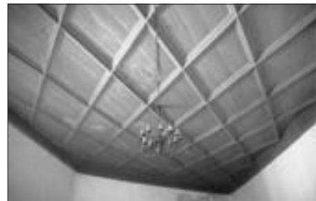
SL. 11. BURG RAPPERSWYL, ŠVICARSKA, PROSTOR NA I. KATU FIG. 11 RAPPERSWYL CASTLE, SWITZERLAND, FIRST-FLOOR
