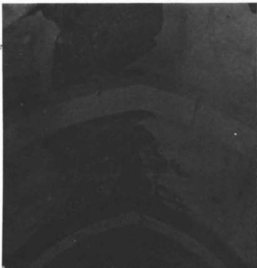
Sl. 2. Gotički svod s dvije pojasnice u crkvi Sv. Luke u Skabrnji. — A Gothic arch with two ribs in the church of St. Luke in Skabrnja
