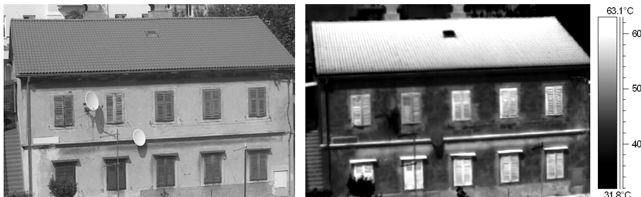
Figure 1. Infrared photo of a building located in the Rijeka's protected urban area (photo taken at 15:30, June 21, 2012)
