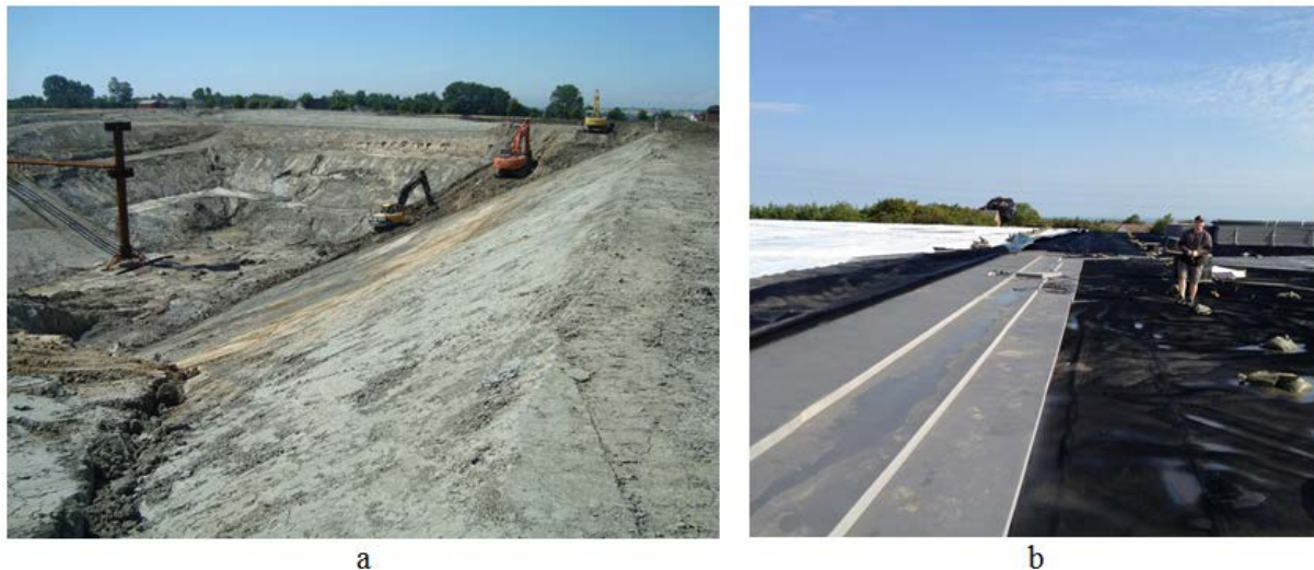
Figure 8. a) Picture of excavation of pit heat storage. The in- and outlet tower is in place and can be seen in the left part of the picture. b) Picture of lid construction of the pit heat storage. The different layers can be seen. In the right part the geo net on top of the liner, in the middle part the three layers of insulation and in the left part another layer of geo net folded back on the white top liner.
