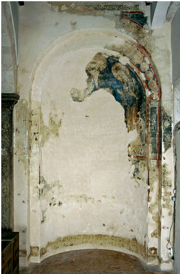
17. Katedrala Sv. Stošije, Zadar, južna apsida, stanje prije radova (fototeka HRZ-a, snimio I. Srša) Cathedral of St. Anastasia, Zadar, southern apse, condition before the works (photographic archive of the HRZ, photo by I. Srša)
