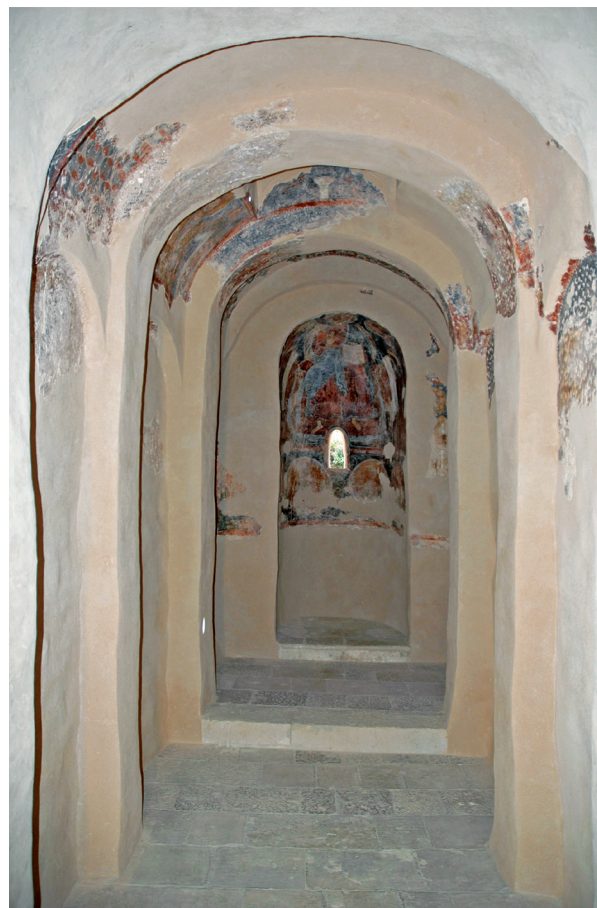
1. Crkva Sv. Ivana, Šilovo selo, stanje nakon radova (fototeka HRZ-a, snimio I. Srša) Church of St. John, Šilovo Selo, the condition after the works (photographic archive of HRZ, photo by I. Srša)
