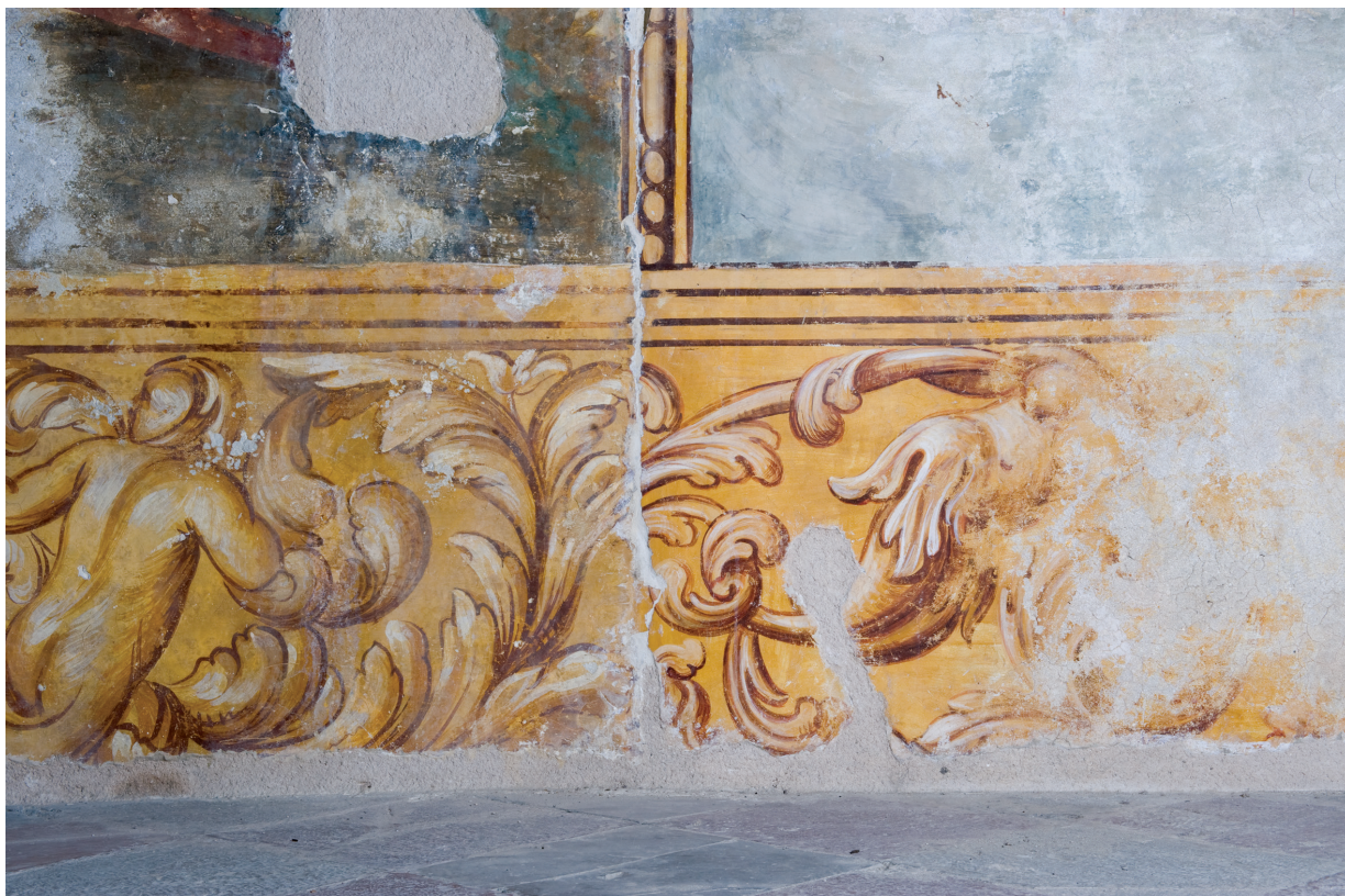
11. Ljetnikovac Sorkočević, južni zid, detalj spoja dvije faze parapeta (fototeka HRZ-a, snimila K. Gavrilica) Sorkočević Villa, southern wall, detail of a join between two phases of the parapet (photographic archive of the HRZ, photo by K. Gavrilica)
