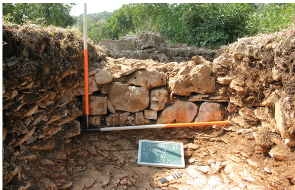
3 Istraženi segment suhozida SJ 26 (fototeka HRZ-a, snimio J. Višnjić) Explored segment of the drywall SJ 26 (photographic archive of the HRZ, photo by J. Višnjić)
