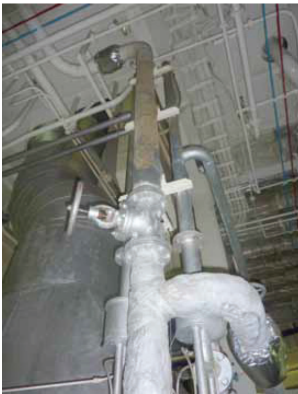
Slika 2. Izolirane cijevi cjevovoda pare Figure 2 Insulated pipes of the steam piping system
