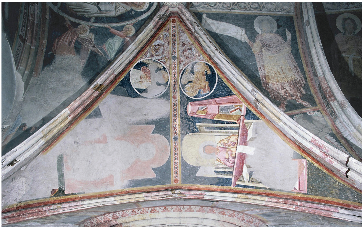
3. Kapela Sv. Stjepana, Zagreb, zapadno svodno jedro, zatečeno stanje (fototeka HRZ-a, snimio V. Barac) Chapel of St. Stephen, Zagreb, southern arch, state found (Croatian Conservation Institute Photo Archive, photo by V. Barac)
