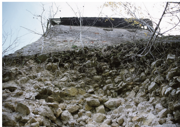
18. Kostajnica, Stari grad, urušenje obrambenog zida ispod peterokutne kule Kostajnica, Old Town, the collapse of the defensive wall below the pentagonal tower
