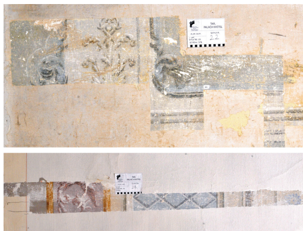
8. Zidni oslik pronaden na zidu i stropu velike dvorane na prvom katu (Fototeka HRZ-a) Wall paintings discovered on the wall and the ceiling in the grand hall on the first floor
