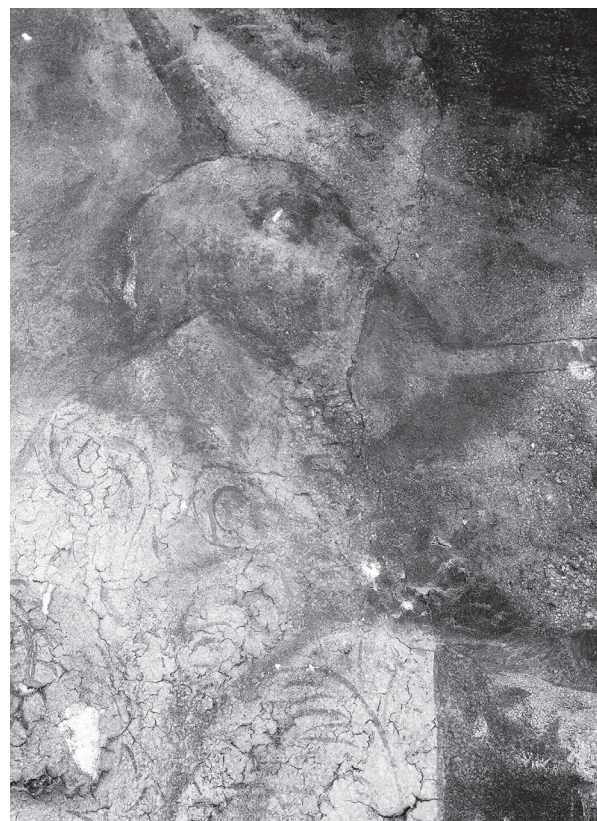
5. Detalj freske na istočnom pročelju crkve sv. Marije, Zagreb, stanje prije restauracije 1972. godine (fototeka HRZ-a, snimila N. Orel) A detail of the fresco on the eastern facade of the church of St. Mary, Zagreb, state before the restoration in 1972 (Croatian Conservation Institute Photo Archive, photo by N. Orel)
