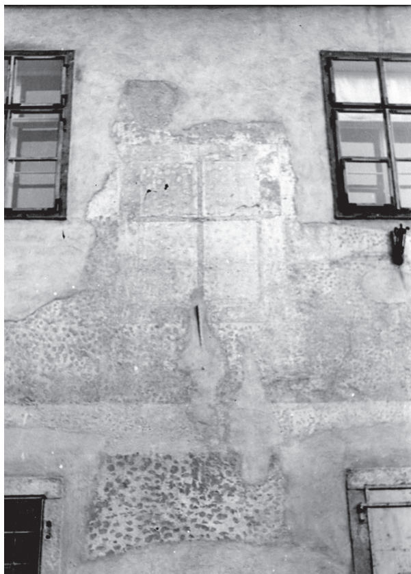
10. Detalj pročelja Muzeja Grada Zagreba, 1954. (fototeka Ministarstva kulture) A detail of the Zagreb City Museum facade, 1954 (Photo Archive of the Ministry of Culture)
