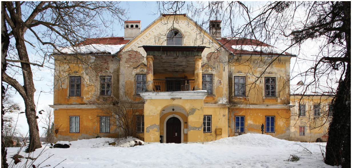
1. Dvorac Jakovlje, pogled prema središnjem krilu dvorca, postojeće stanje (snimio Z. Bogdanović) The Jakovlje Mansion, view to the central wing of the mansion, current condition (photo by Z. Bogdanović)
