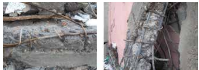
Figure 29. Poor hook arrangements at the end of lateral confinement bars
