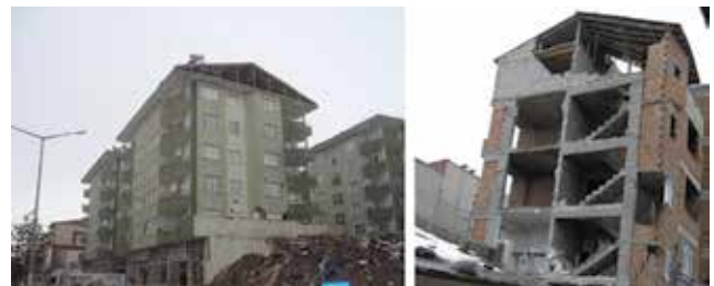
Figure 18. Out-of-plane deformation damage of the gable walls
