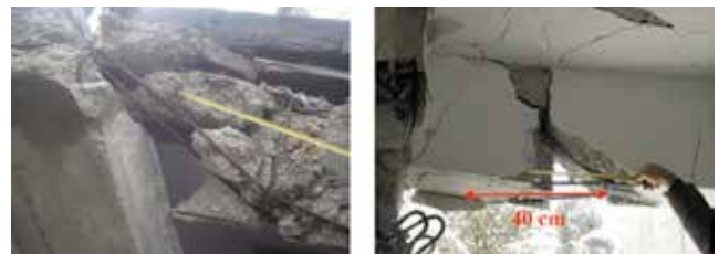
Figure 28. Inadequate lateral reinforcement intervals
