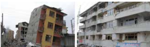
Figure 12. Collapse of two buildings due to soft storey effect at the ground floor level in Erciş
