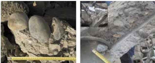
Figure 25. Inappropriate aggregates used in Reinforced concrete buildings
