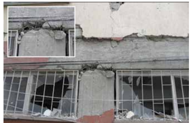
Figure 13. Shear failure at the top of the column due to short shear span in Van
