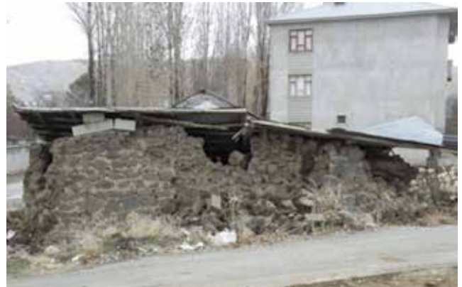
Figure 22. Collapsed masonry building due to the lack of connection and mortar on the walls and roof in Erciş
