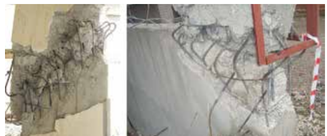
Figure 30. Shear damage and buckling of longitudinal reinforcement due to insufficient lateral rebar interval
