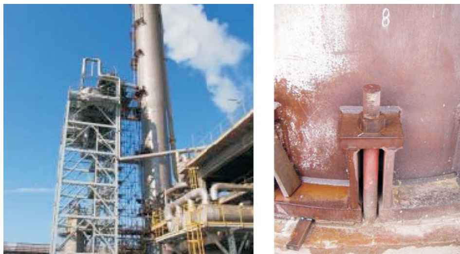
Fig. 1. The desorbing tower (left) and the anchorage of the tower on the foundation (right).
