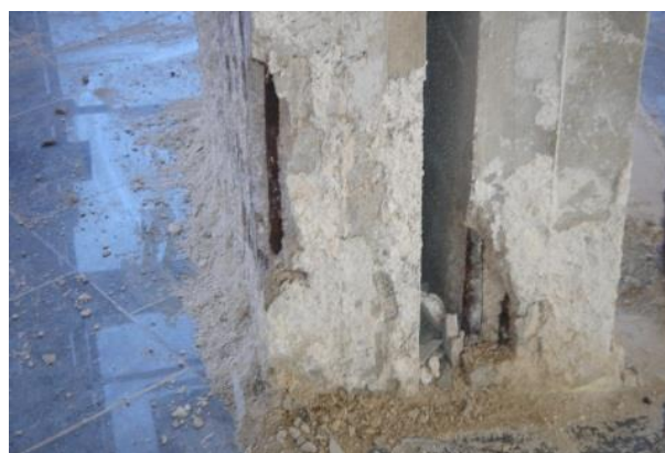
Figure 1. Examples of types of damage noticed in old buildings
