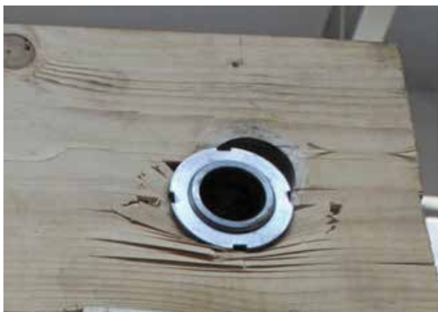
Figure 10. Deformation of edge joint in the second truss
