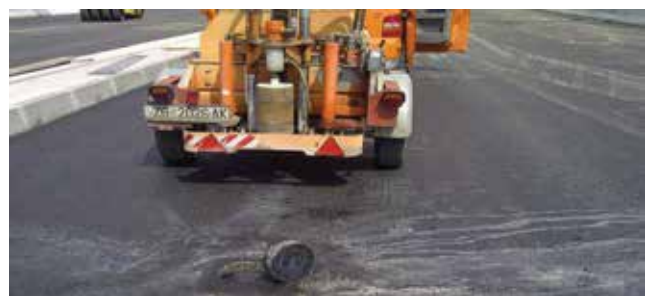
Figure 7. Sample taken at the Odra Viaduct from the completed waterproofing – asphalt system
