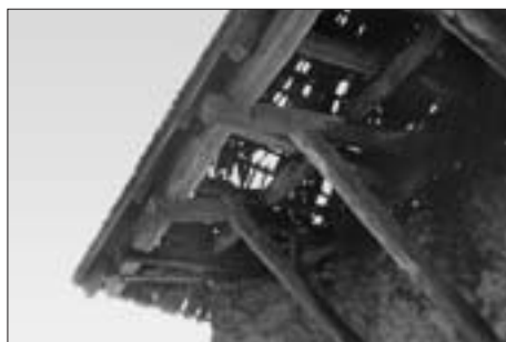
SL. 12. OZALJ, PALAS KNEZOVA FRANKOPANA I ZRINSKIH ZVAN „ŽITNICA”: JUGOZAPADNI UGAO S KARAKTERISTIČNOM SNAŽNOM STREHOM FIG. 12 OZALJ, FRANKOPAN AND ZRINSKI'S PALACE, CALLED „GRAINSTORE”: SOUTH-WEST CORNER WITH ITS TYPICAL STRONG EAVES
