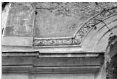
SL. 8. RAŠCLAMBA VANJSKIH ZIDOVA CRKVE U PLAŠKOME FIG. 8 OUTSIDE WALLS OF THE PLAŠKI CATHEDRAL
