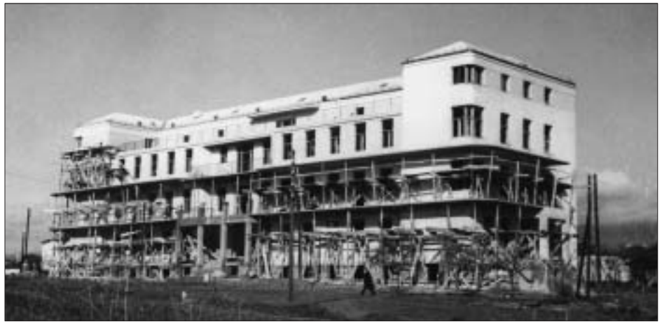
SL. 8. IZGRADNJA ORTOPEDSKE I ZUBNE KLINIKE, 1931. FIG. 8 ORTHOPEDIC AND DENTAL CLINICS, CONSTRUCTION, 1931
