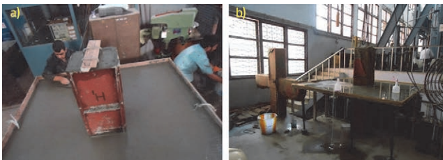
Figure 4. Construction of test specimens: a) Casting of the test specimen JS; b) Curing of the test specimens
